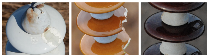
Figure 1: Flashover damage, Broken and Good class examples
